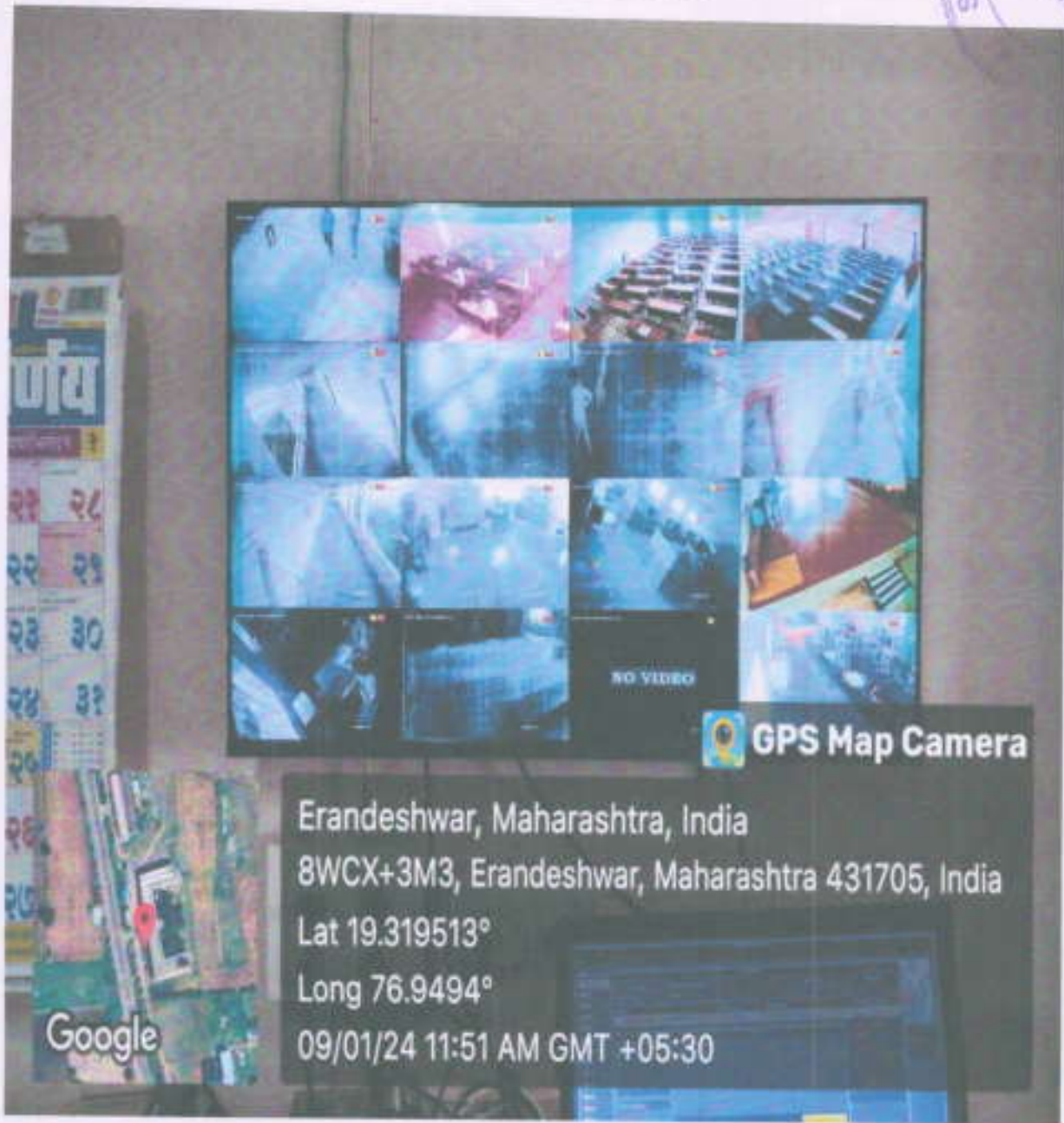
CCTV CAMERA SLIDES AT PRINCIPAL CABIN
